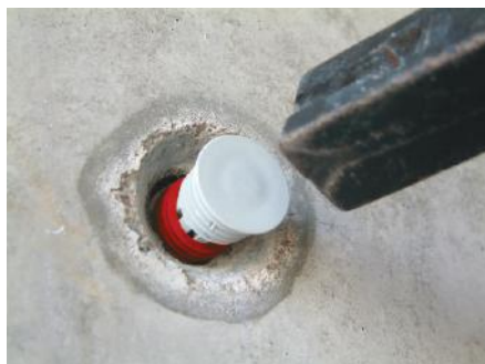
2. Hammer the Solco Form-Tie Plug with light blows from a hammer until flush with the end of the conduit sleeve
